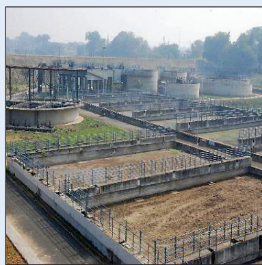
Treatment Plant, Varanasi
